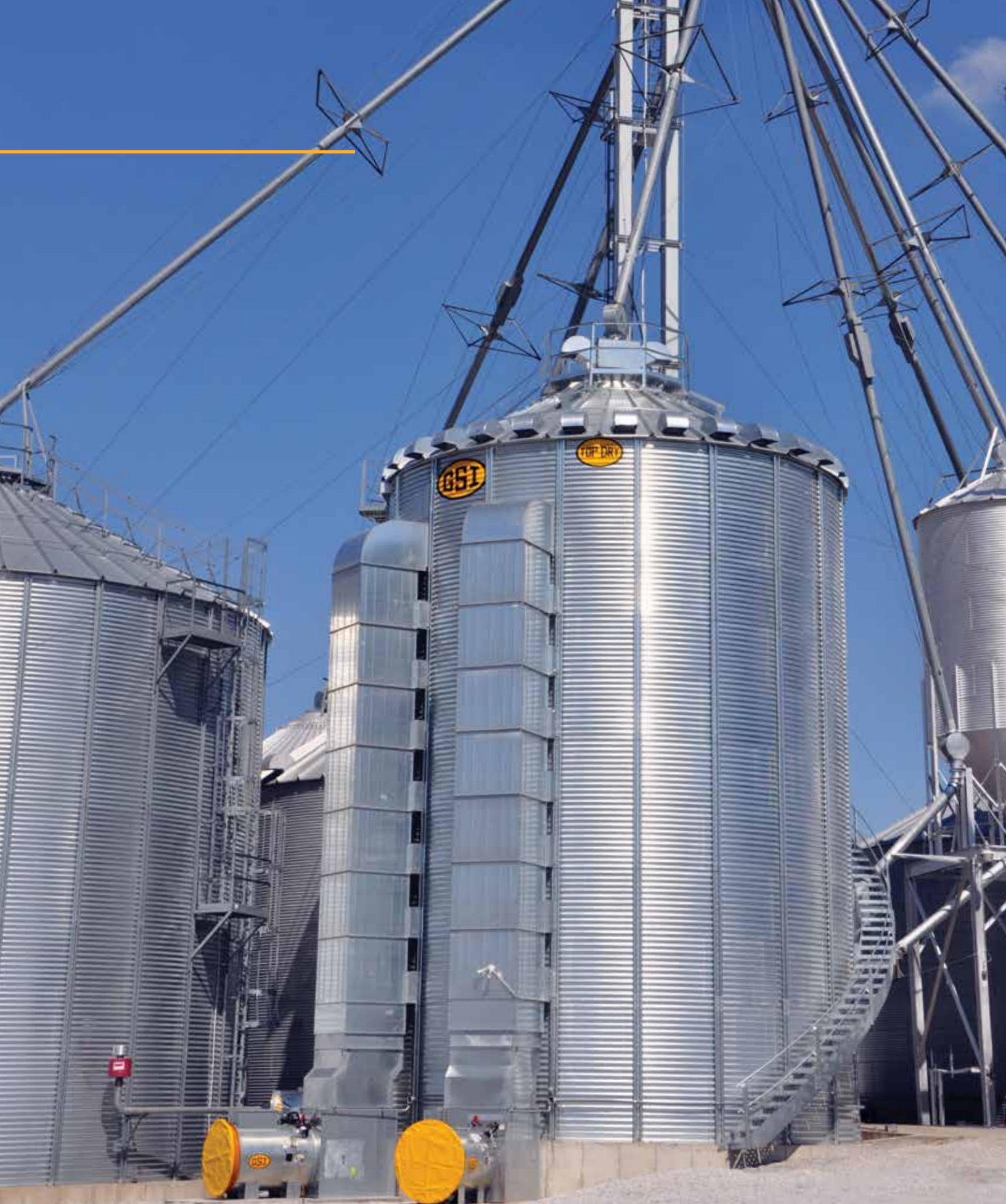
Dealer supplied offset to ductwork for taller foundation.
